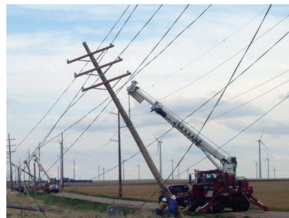
Downed power lines like this one had to be repaired to restore power.
