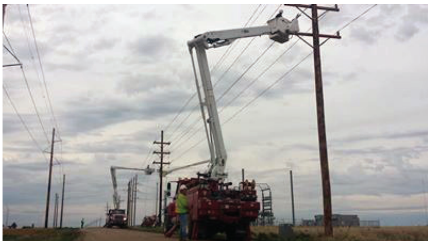
Line crews safely repair lines to restore power back to more than 6,000 members.
