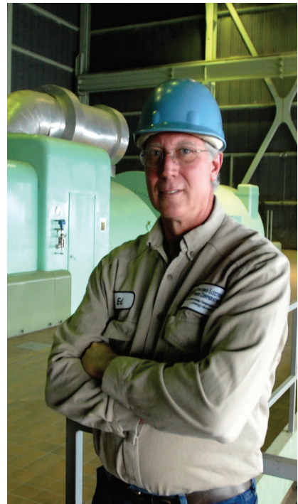
Ed Eversole, Sunflower, stands with a natural gas unit at the Fort Dodge Station.
