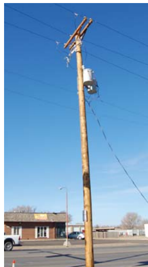
To complete the process, the transformers are attached and hooked into the phases above. The temporary transformer that was installed is removed and power flows normally again. This whole process allows the linemen to work safely and members to maintain power.
